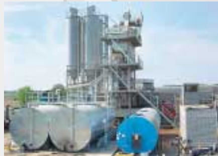
Vertical filler storage system and horizontal bitumen tanks
