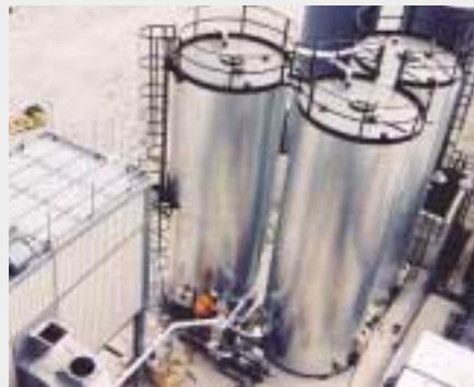
Vertical bitumen storage system
